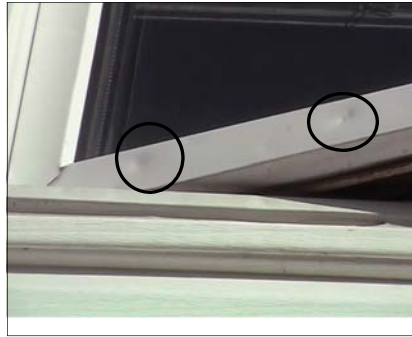
Denting of window sashes, wraps and frames can be barely visible. Use your fingertips to feel the dents.
