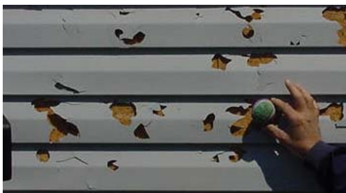
Cracked and perforated vinyl siding. In light hail areas small cracks can look like a strand of hair and can be hard to see. Wood siding may need to be repainted or re-stained.
