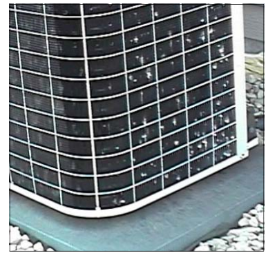
Damage to air conditioner fins reduces cooling efficiency.
