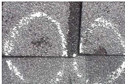
Denting and fracturing of shingles can be more evident after winter.
